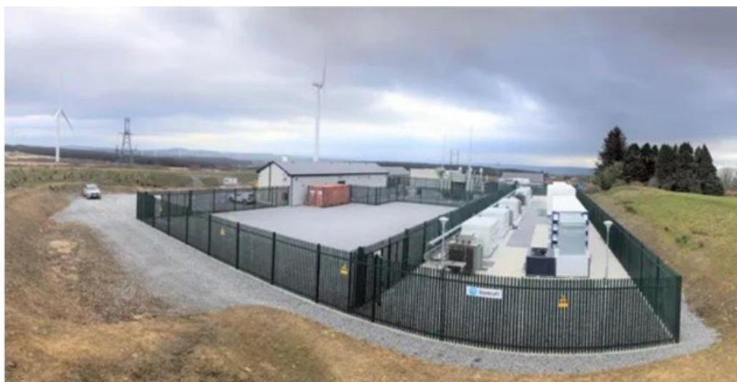
Statkraft's battery park in Kilathmoy, Ireland.
