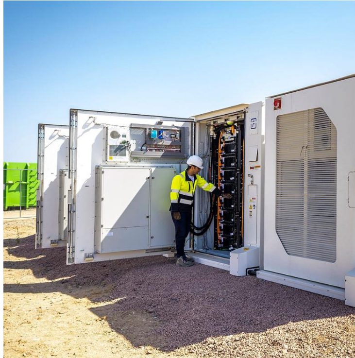
Europe 15: wind, solar, BESS and grid
